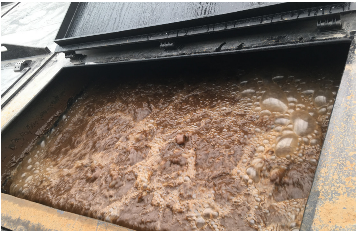
Figure 2 Wastewater tank with BIO-CEL® L-1 modules installed
