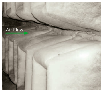
Filtres Tri-Dek® RFX installés
