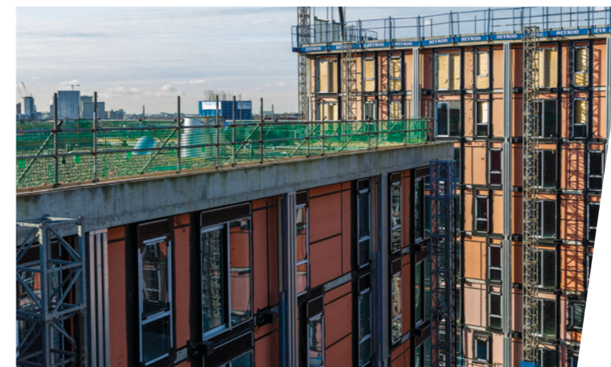
Knauf Windliner installed on Middlewood Locks mixed-use development in Salford, Greater Manchester
