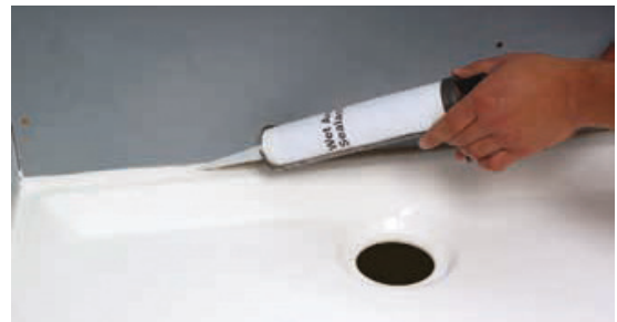
Figure A11: Seal Sheet Edges Over Baths, Shower Bases, and Laundry Tubs
