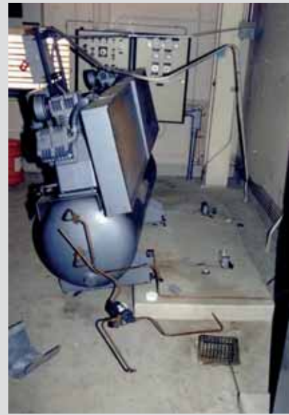
b) Sliding of a compressor without seismic restraints, 1994 Northridge Earthquake, Los Angeles, USA /Wiss, Janney, Elstner Associates, Inc/
