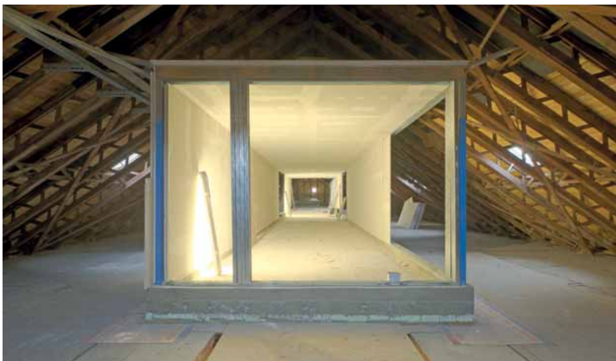
Fig. 3.22: A 31.5 m long and 3.65 m wide Cubo construction in fire-resistant design in the attic for subsequent installation of the complete ventilation equipment in the old local court building in Offenbach (during installation) /Knauf Gips KG/
