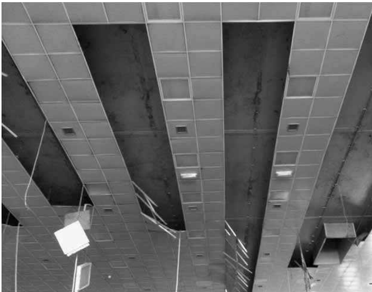
Fig. 4.33: Failure of a large suspended lightweight steel gypsum board ceiling, 2012 Emilia Earthquake, Mantova, Italy /Marco Savoia/
