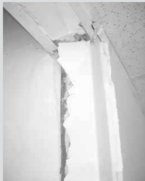
b) Damage at joints between steel structure and a lightweight gypsum board partition, Knauf De Chile Ltda Offices, 2010 Chile Earthquake /Knauf Chile/
