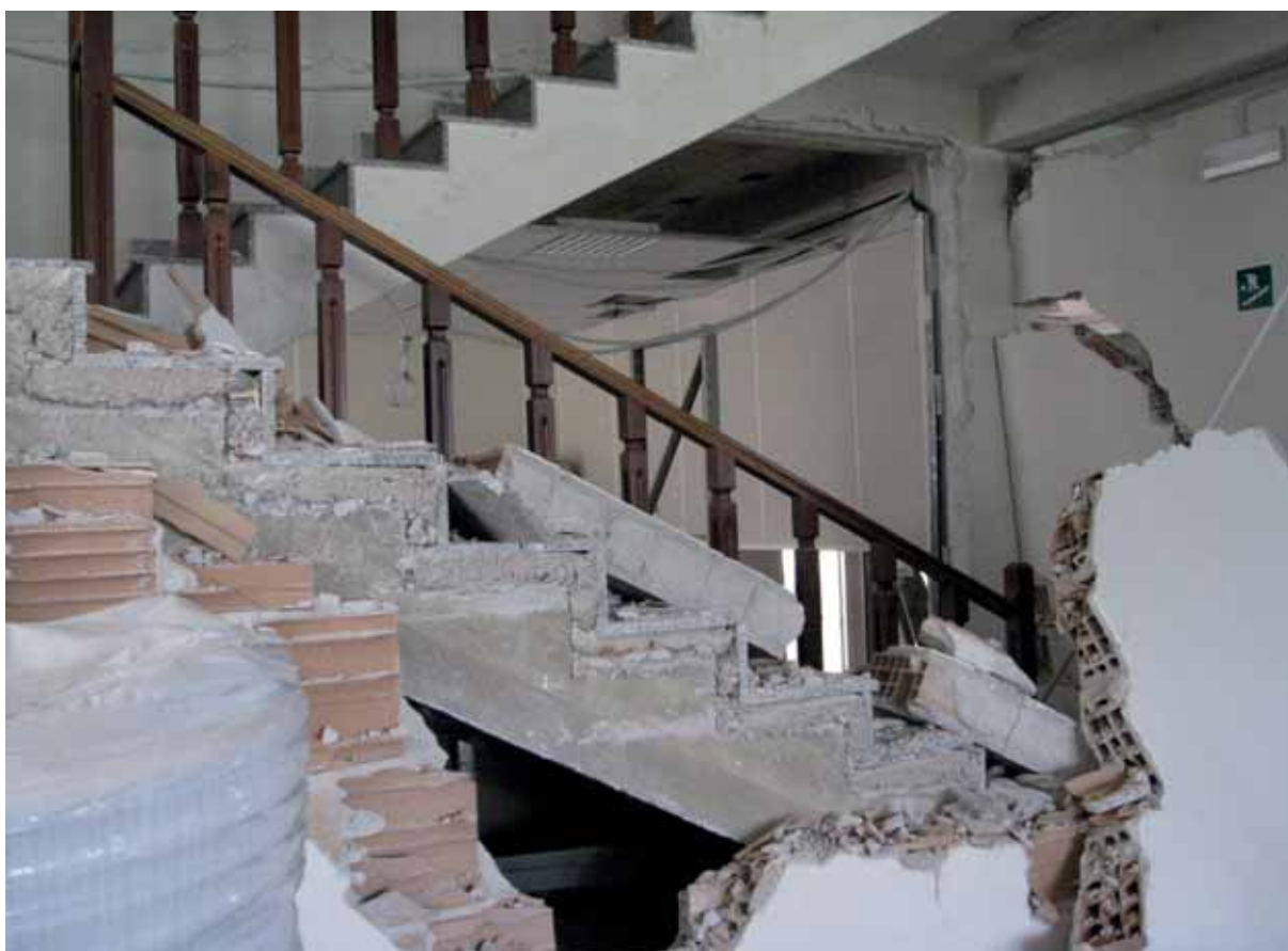
Fig. 4.2: Collapse of non-structural components in a storehouse, 2009 Abruzzo Earthquake, L'Aquila, Italy
