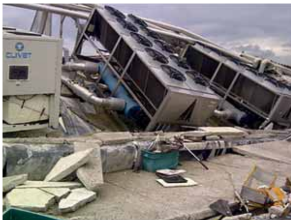
Fig. 4.36: Functionality loss risk: Damage to essential services in a biomedical company, 2012 Emilia Earthquake, Medolla, Italy /Marco Savoia/
