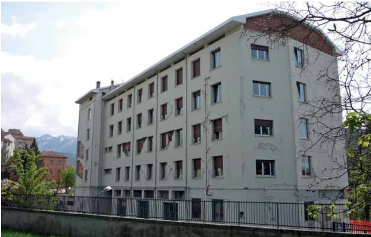
Fig. 4.4: Damage to non-structural components in a public building, 2009 Abruzzo Earthquake, L'Aquila, Italy
