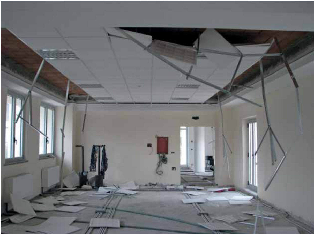
Fig. 4.34: Life safety risk: Damage to non-structural components, 2009 Abruzzo Earthquake, L'Aquila, Italy /Angelo Masi/
