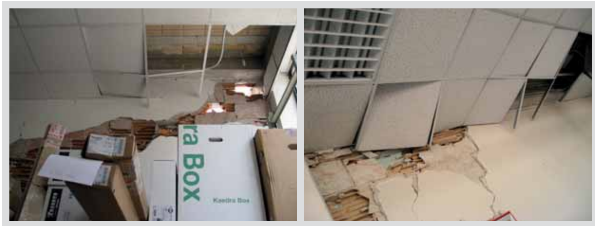
Fig. 4.31: Damage to suspended acoustic lay-in tile ceilings, 2009 Abruzzo Earthquake, L'Aquila, Italy
