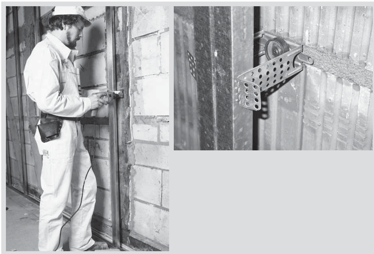
Fig. 3.9: Directly anchored furring with formation of the coupling point to the basic wall /Knauf Gips KG/
