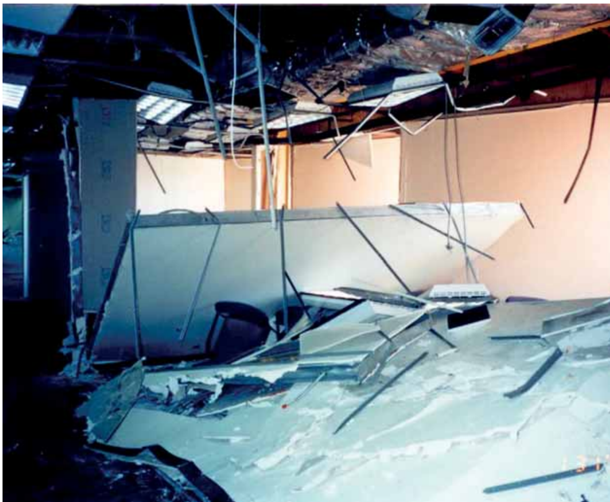
Fig. 4.30: Out-of-plane failure of an unbraced partial-height lightweight steel gypsum board partition due to the inertial forces, 1994 Northridge Earthquake, Los Angeles, USA /Wiss, Janney, Elstner Associates, Inc./
