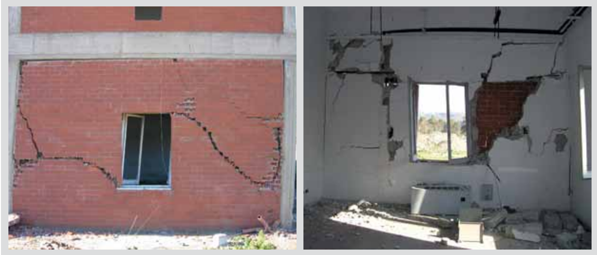
Fig. 1.1: Earthquake damage of traditional constructions
