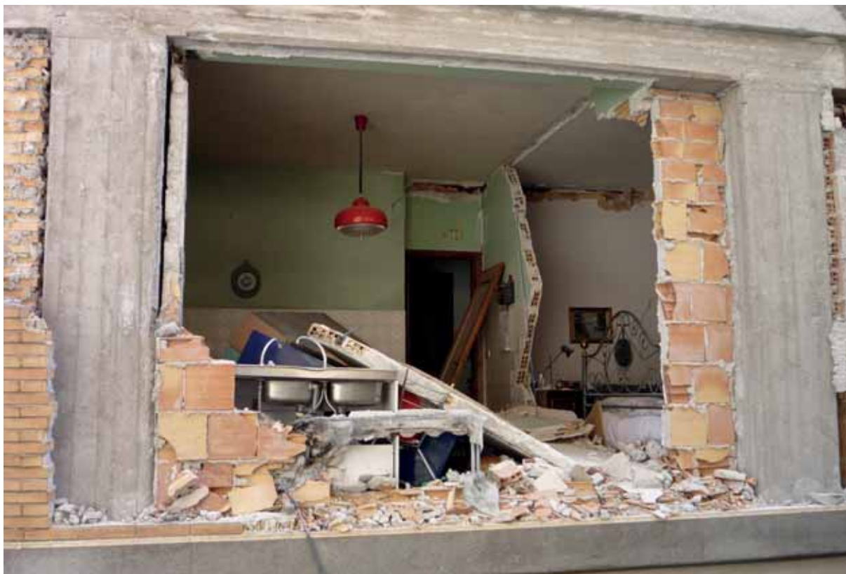
Fig. 4.1: Collapse of non-structural components in a residential building, 2009 Abruzzo Earthquake, L'Aquila, Italy
