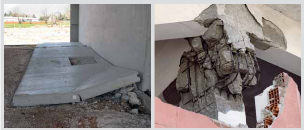
Fig. 1.2: Earthquake damage of traditional constructions
