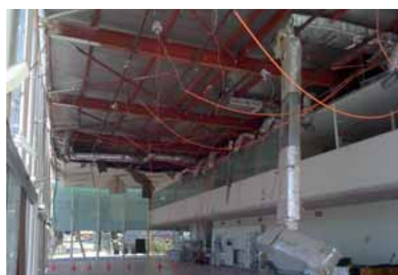
Fig. 4.28: Effects of the interaction between non-structural components and systems: Collapse of a suspended lightweight gypsum board ceilings due to the presence of a heavy HVAC ductwork in a commercial building, 2010 Chile Earthquake /Knauf Chile/
