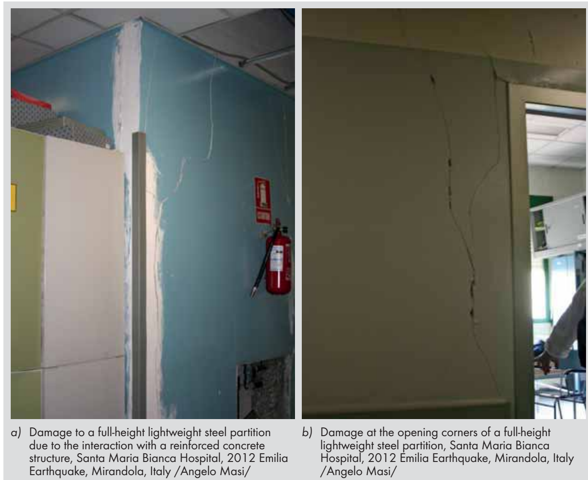
Fig. 4.29: In-plane damage to lightweight steel gypsum board partitions due to the building deformations
