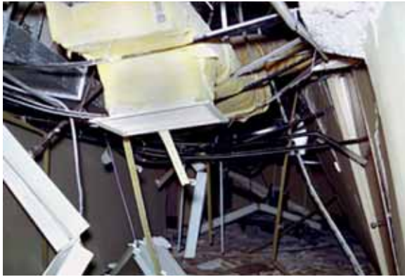
Fig. 4.37: Damage to non-structural components at the Olive View Medical Treatment Building, 1971 San Fernando Earthquake, Los Angeles, USA /NISEE-PEER/
