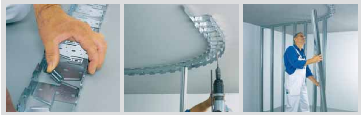
Fig. 3.31: Walls with radii from 125 mm with profile Sinus, Knauf system /Knauf Gips KG/
