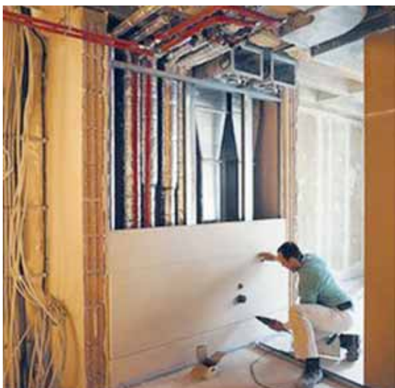
Fig. 3.10: Installation shaft wall design, Knauf system W628, Type A /Knauf Gips KG/
