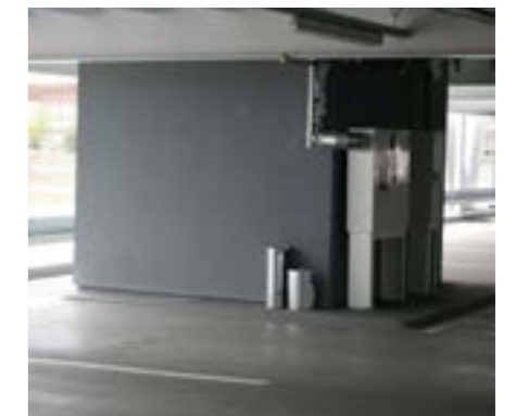
Car Park Utility Rooms | Stuttgart, Germany
