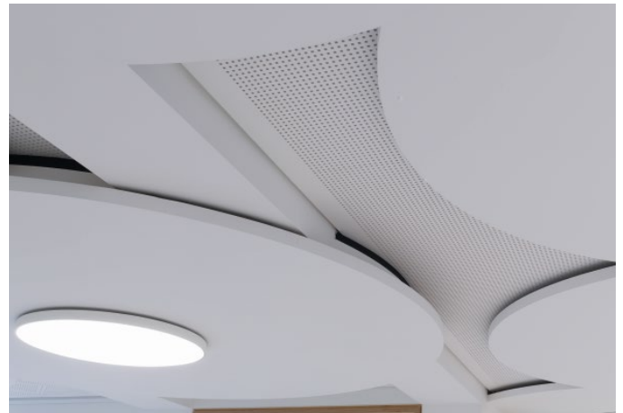
The new ceiling is arranged in three levels in height and cover the relatively low set reinforced concrete beams as well (Photo: Knauf/Clemens Ortmeier).
