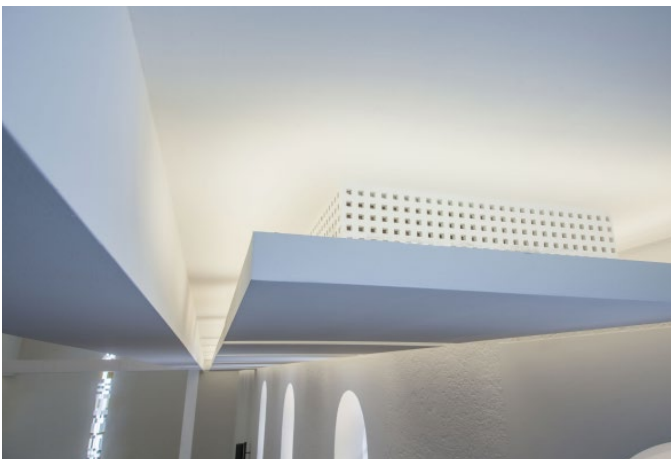
Ceiling canopies made of Knauf Tectopanel acoustic plaster base boards with acoustical plaster absorb the sound in the church.
