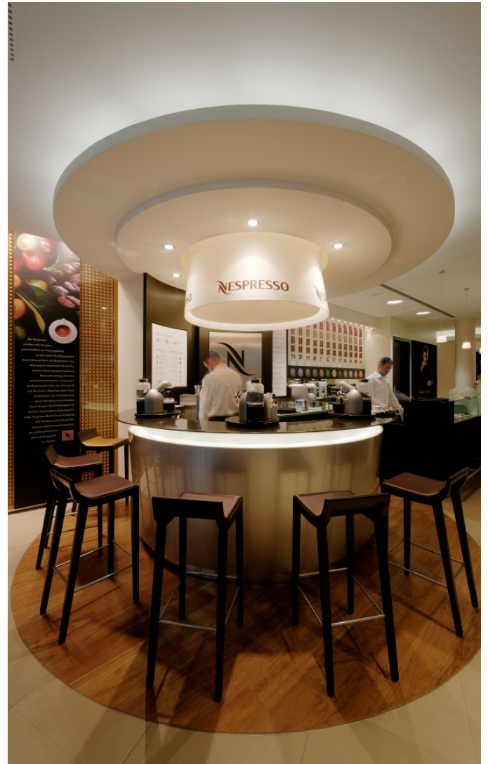
Ceiling construction of the shop - The ceiling is suspended via many layers, the lighting is integrated and plastered in.
