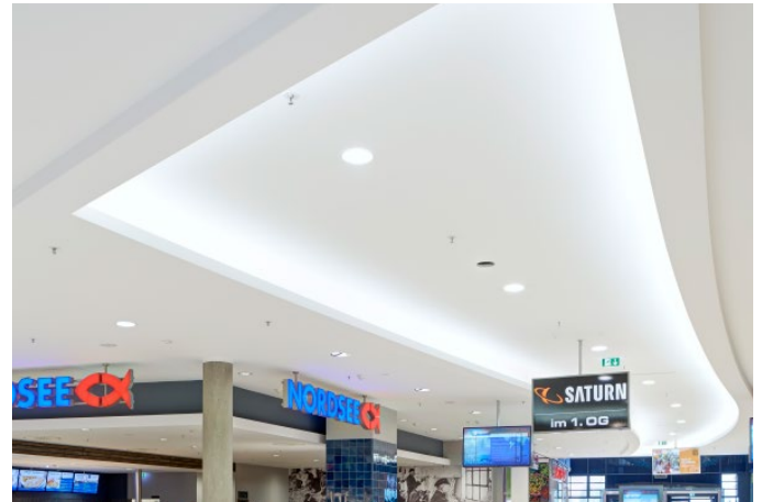
Recessed ceiling levels with recessed lighting guides the visitor and aptly puts the shopping arcades in the limelight. More than 2500 linear metres of L design units were installed.
