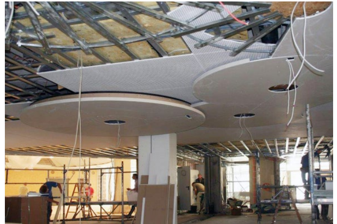
Ceiling construction of the foyer with the three ceiling levels during the building phase. (Photo: Jaeger Ausbau)
