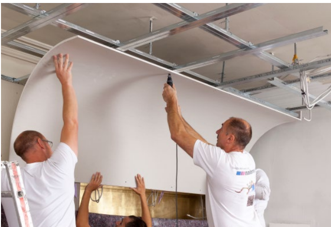
The drywallers manufacture the ceiling canopy above the seating niches in the lounge from prefabricated boards to reduce the assembly time.
