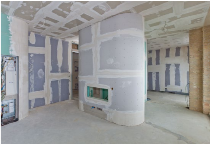
Drywalling know-how from Knauf forms the basis, and not just for the curvaceous room designs.
