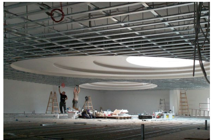
Detail of the ceiling construction in the Max-Planck-Institute. (Photo: Ruben Peter Ausbau GmbH)
